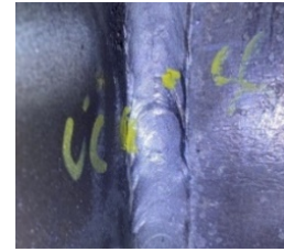
Figure 3. Undercut Defect (source: PT. INKA Multi Solusi)
