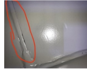
Figure 4. Overlap Defect (source: PT. INKA Multi Solusi)
